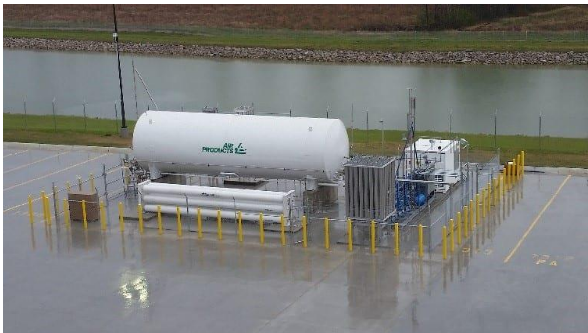
Figure 7: Hydrogen Fueling Equipment Example
